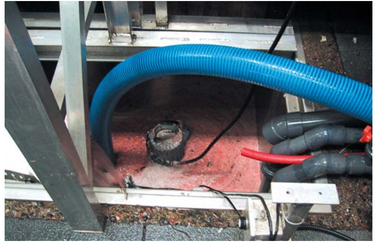
Ground floor waste sump using Flygt NS-3102
