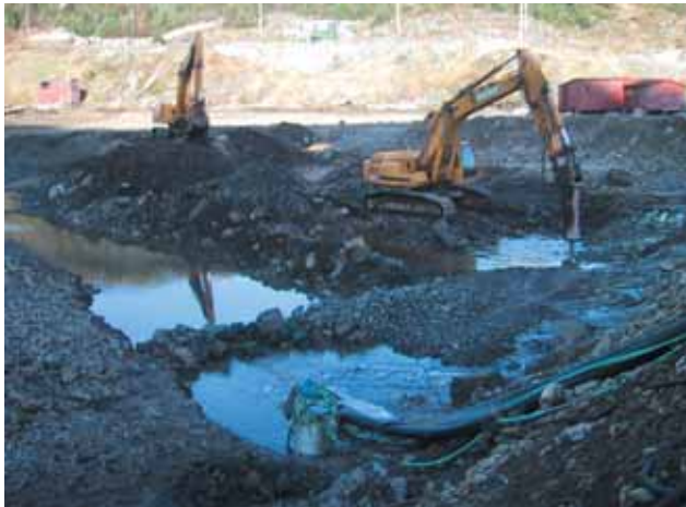
The dredging site where we can see Flygt BIBO pumps in the foreground.
