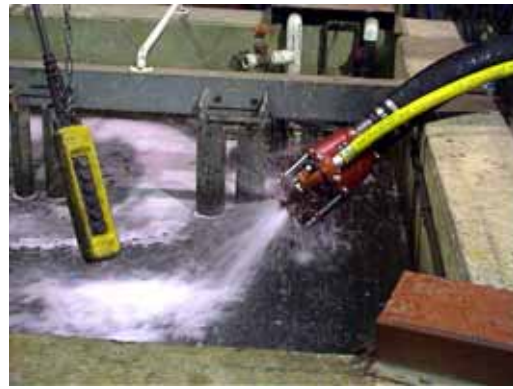
Fig. 2: Suction line during priming
