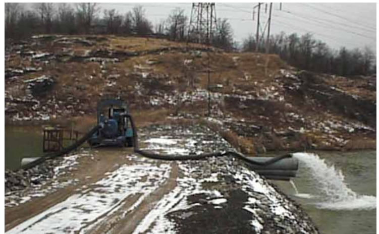
Fig. 1: The Thompson 6-inch Compressor-Assisted Dry-Prime pump recirculated the acidic water and lime mixture to maintain pH levels and made the water safe to return to the environment.
