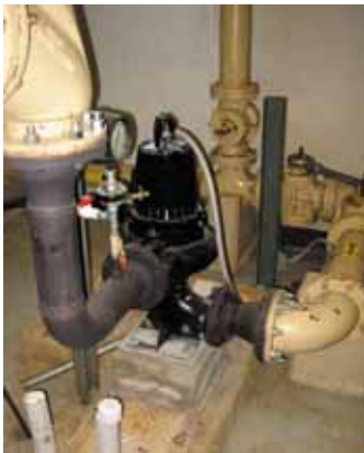
Sludge loading pump.
