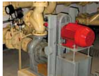
Old sludge loading pump similar to the one replaced.
