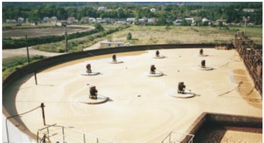
Surface movement in the aeration basin, Cell #2, approximately five minutes after the aerators were turned off.
