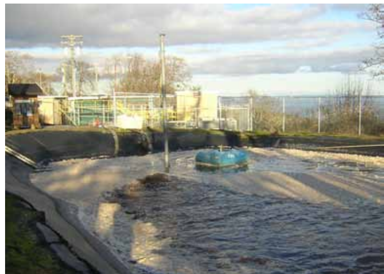
The temporary lagoon where the Flygt Jet Aerator, the N 3153 submersible pump and the flotation module were installed.
