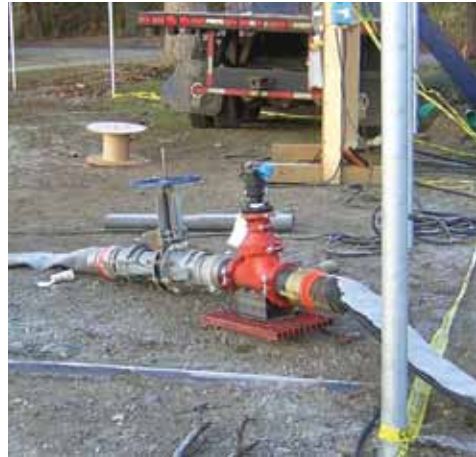
The combination valve (vacuum breaker & air release) and a 6" gate valve to manage the flow.
