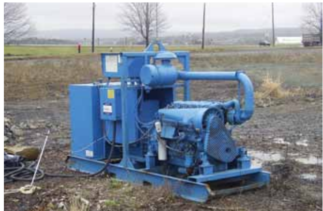
12" Kwik-Lok steel galvanized piping and a Flygt 100kW generator.
