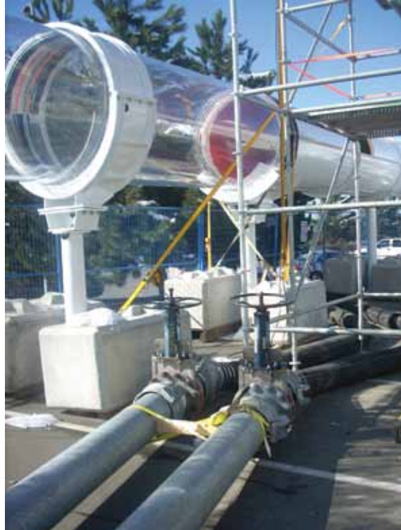
12" knife gate valves to control the flow shown here.
