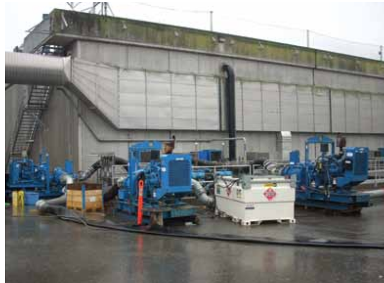
Skid-mounted ENVIROPRIME® Diesel Driven Thompson pumps and fuel tank.
