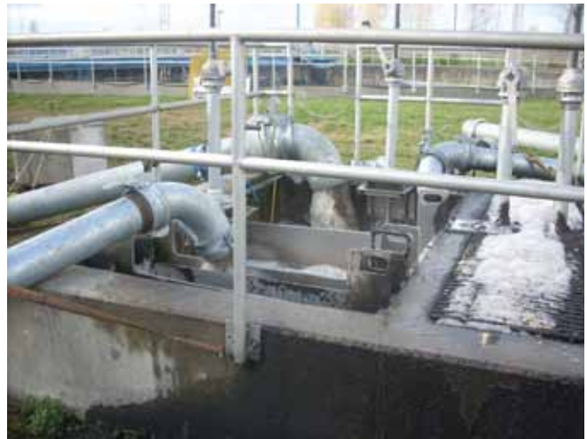
12 inch Kwik-Lok steel piping discharging bypassed sewage.
