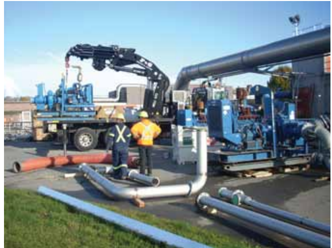
Unloading of Thompson Diesel Driven pumps and assembling of discharge pipes on site.
