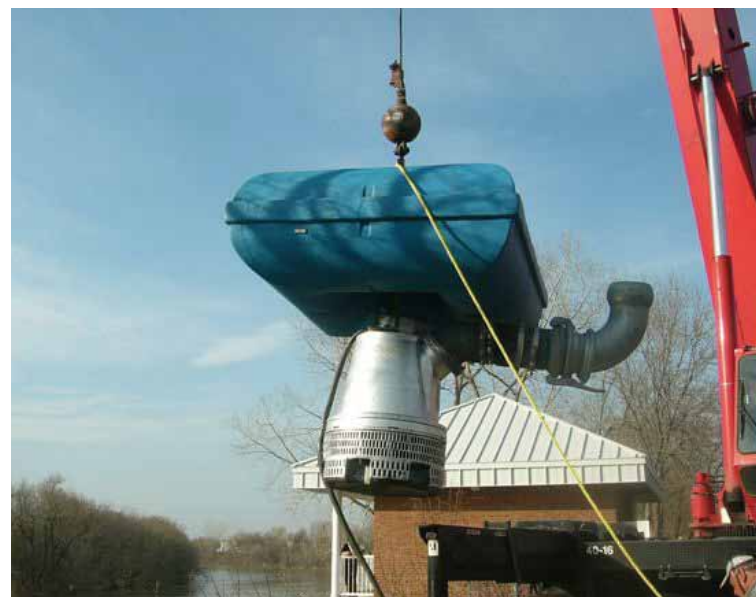
1150 PFM flotation module and the BS 2250 Flygt pump in the process of being installed.
