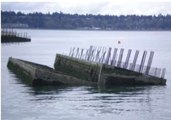
One of the 6 partially sunken caissons damaged during a storm.
