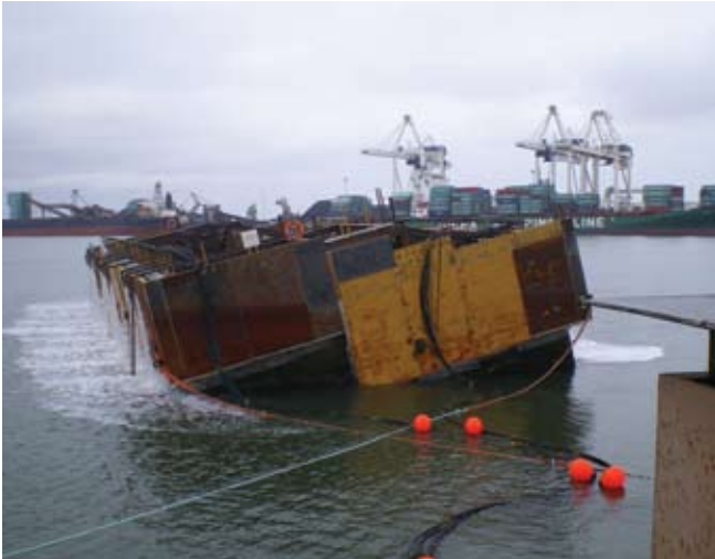
The power cables were bundled together and attached to buoys.
