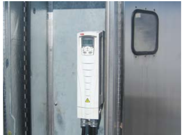
Flygt ACS550 Variable-frequency drive (VFD).
