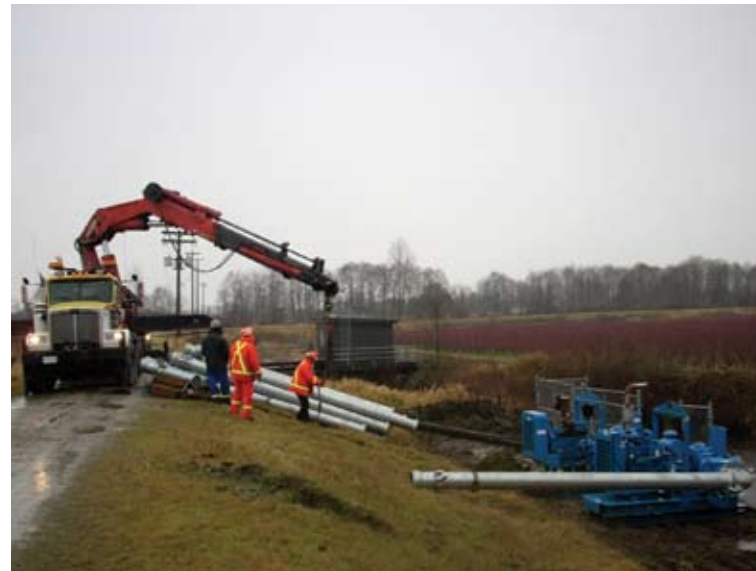
A mobile crane was called on the job site to install the diesel driven pumps and piping discharge connections.
