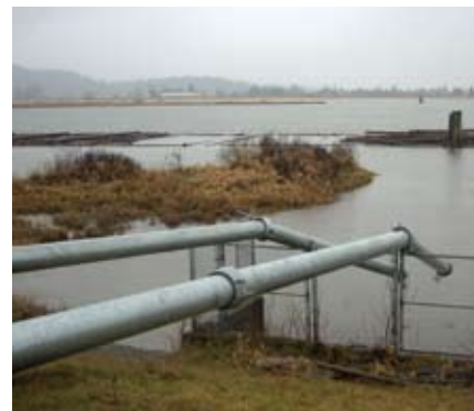
The 2 piping discharge connections overlooking the Fraser River.
