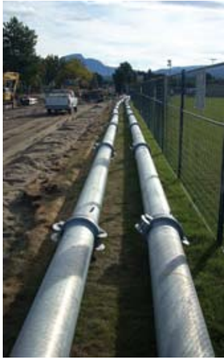
12 in. steel piping on site
