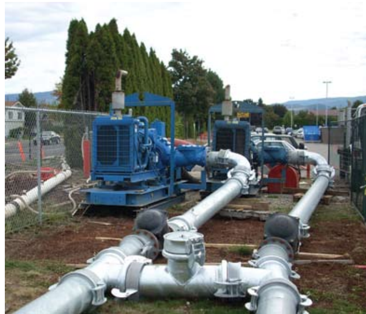
Diesel driven pumps, check valves and steel piping were used in this bypass.
