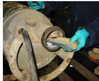
Hardened "back fill" material left behind - removed while servicing the pump.
