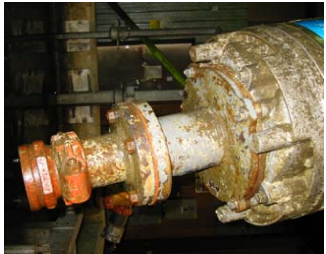
The tandem connection fabricated by the Flygt Sudbury sales location required for connection to the transfer tank.
