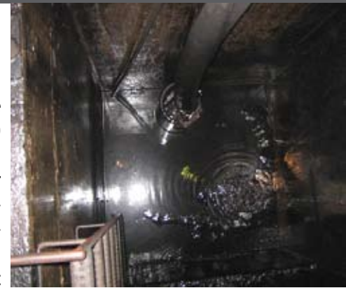
Floor wash down sump
