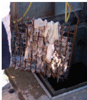
One of the screens collecting solid materials from getting into the wet well.
