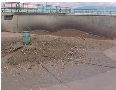
Note freeboard. Low levels were maintained in an effort to contain overspray from surface aerators. This was not always successful.
