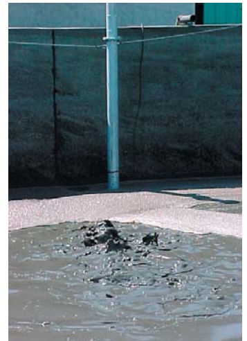
Air bubbles rising from Jet Aerator.
