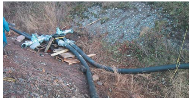
The check valves and by-pass gate valves are installed just above the beach near the generator.
