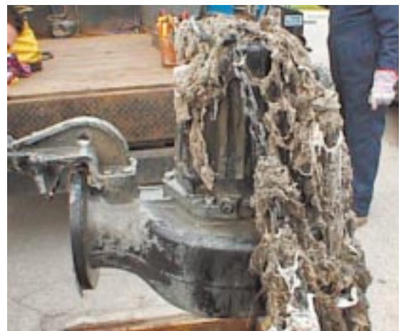
Figure 6. ITT Flygt N-pump after three months of operation at the Ste-Thérèse field test station.
