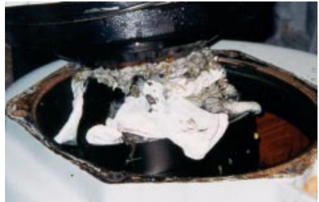
Clogged impeller of the regular pump, during trial period.
